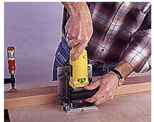
5--To cut plate slots in the panel's center, clamp a fence across the panel to guide the vertically positioned plate joiner.
